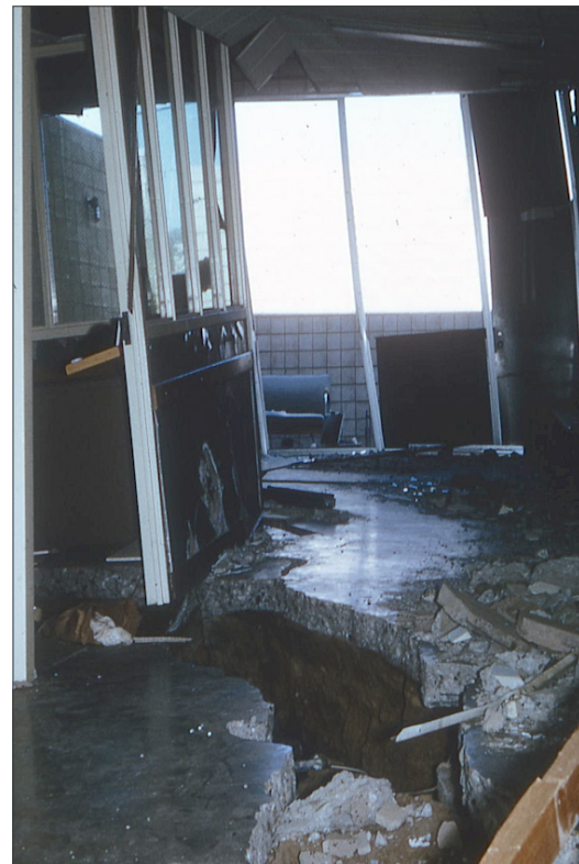
Figure 13. View of interior of building pulled apart by liquefaction-induced lateral spread at San Fernando Juvenile Hall during the 1971 San Fernando, California earthquake. Photo by T.L. Youd.
