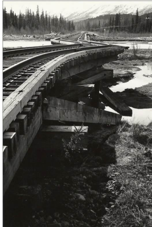
Figure 12. View of railroad bridge compressed by liquefaction-induced lateral spread during the March 23, 1964 Alaska earthquake. Photo courtesy of the U.S. Geological Survey.
