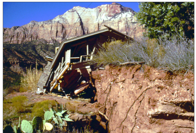
Figure 24. Damage to a home caused by the Springdale landslide in the 1992 M 5.8 St. George earthquake.
