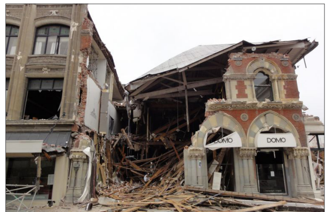
Collapse of URM building - 2011 Mw 6.1 Christchurch, New Zealand earthquake. Photo: EERI/Justin Marshall.
