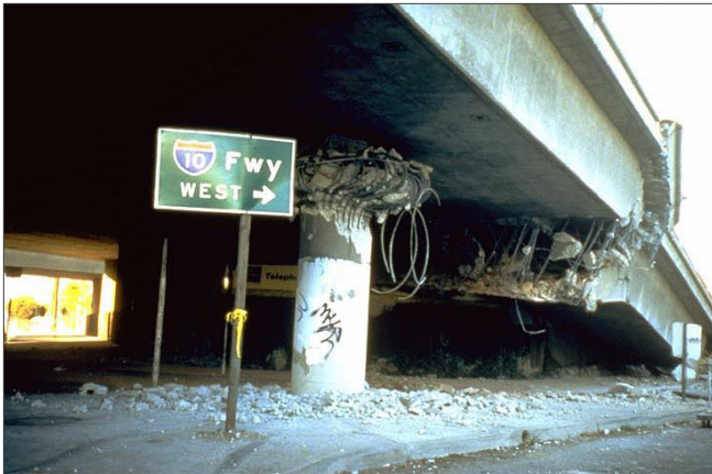
These non-ductile columns failed in shear and then collapsed under the weight of the bridge - 1994 M_w 6.7 Northridge, California earthquake. Photo: EERI.
