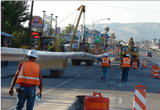
Installation of a welded steel natural gas pipeline in Salt Lake County. Photo courtesy of Quester Gas Company.
