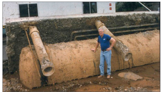
Figure 18. Buried oil storage tank at an industrial facility that floated to ground surface due to liquefaction of subsurface soils during the 1993 Hokkaido-nansei-oki, Japan earthquake. 24
