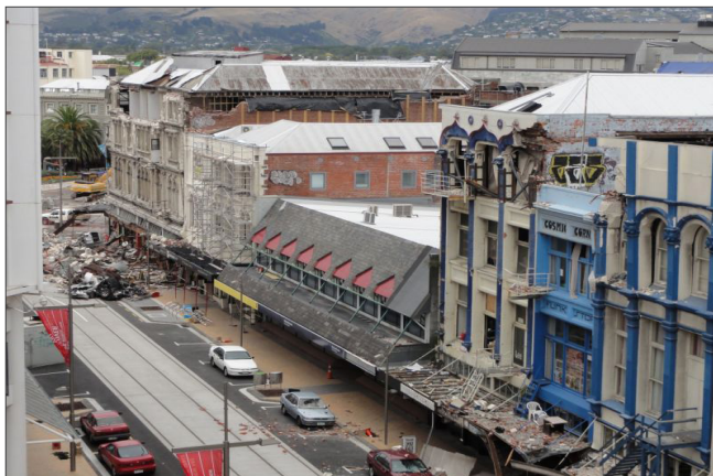
Damage to Central Business District. Mostly collapse of URM - 2011 Mw 6.1 Christchurch, New Zealand earthquake. Photo: EERI/Mary Comerio.
