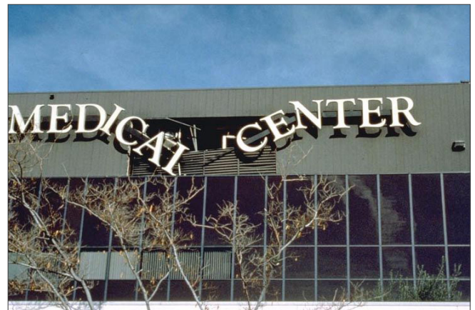
HVAC service outage at the Holy Cross Medical Center in Sylmar caused evacuation of all patients. The damage shown occurred when suspended fans in the penthouse swung and impacted louver panels. This building, a steel frame, also suffered many weld fractures that were not discovered until well after the facility had been restored to service - 1994 M_w 6.7 Northridge, California earthquake. Photo: EERI.
