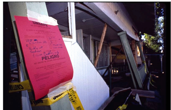
Detail of unsafe posted single family dwelling unit - 1994 M_w 6.7 Northridge, California earthquake. Photo: EERI
