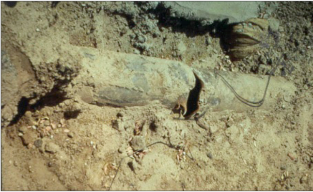
Figure 14. View of water pipeline rupture due to liquefaction-induced lateral spread near the San Fernando Juvenile Hall during the 1971 San Fernando, California earthquake. Photo by T.L. Youd.
