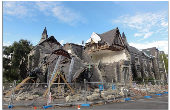
Collapse of URM church - 2011 Mw 6.1 Christchurch, New Zealand earthquake. Photo: EERI/Justin Marshall.
