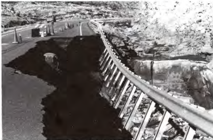
U. S. Highway 191 damage with the water gap to the right. Note the shallow channel which normally carries runoff without overflow (photo by Paul Guardy).
