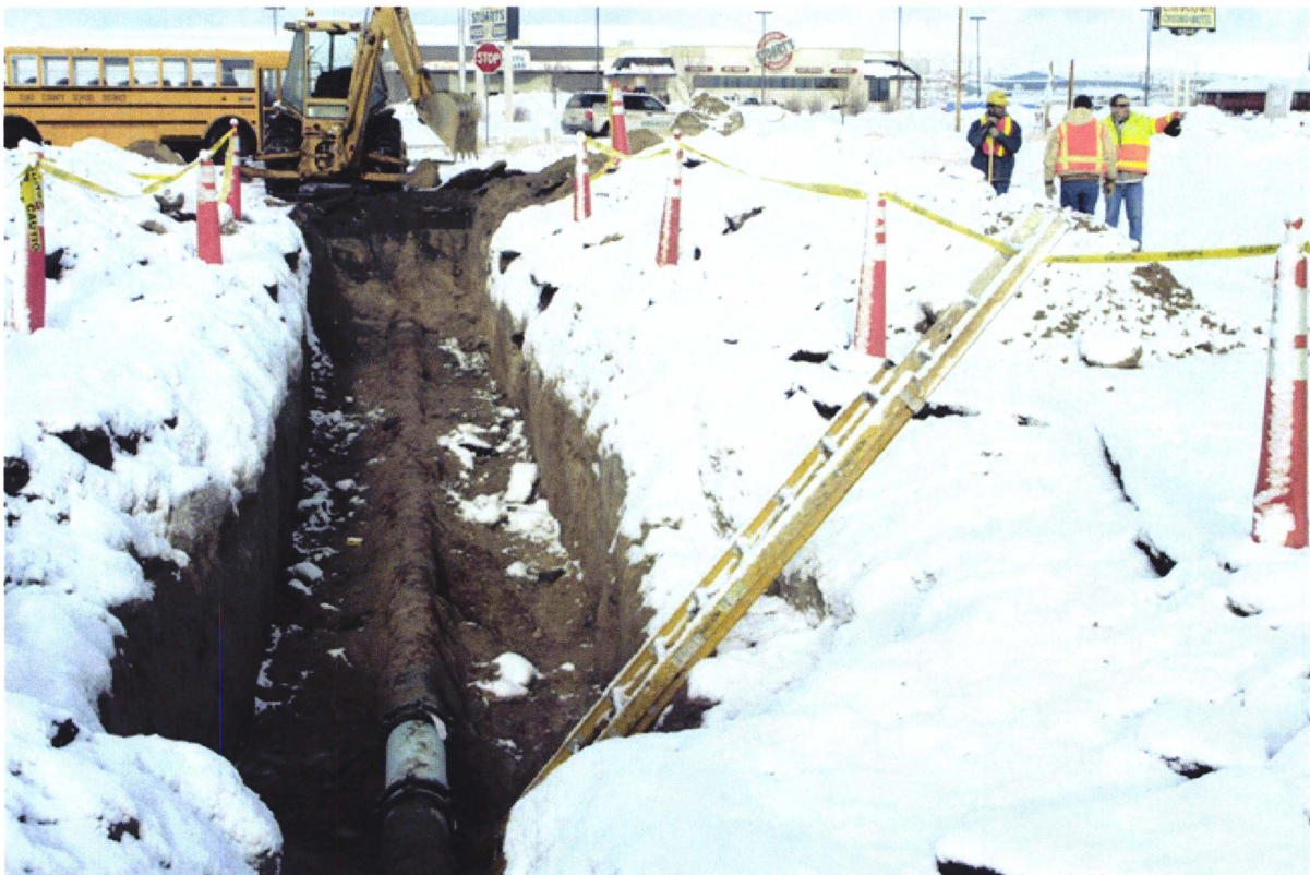
Photo 2. Water main break in Wells.
