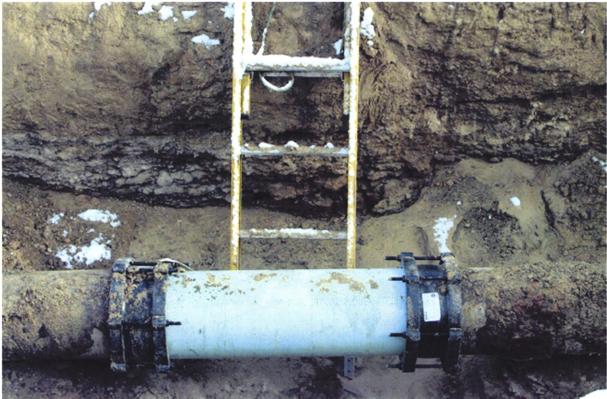
Photo 3. Water main break in Wells.
